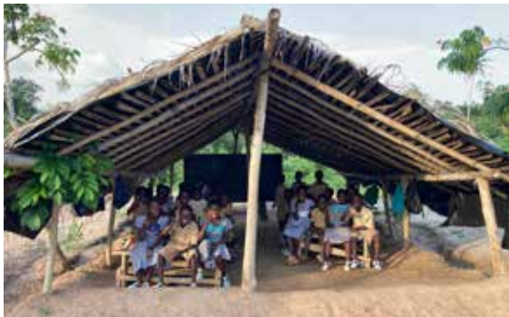
One classroom in N'zidrikro primary school before the works
